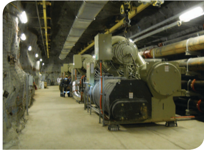
Custom built for reliability under extreme conditions, Trane CenTraVac chillers help to keep mine workers comfortable.
