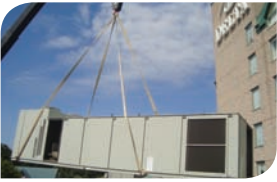
The Trane IntelliPak II™ rooftop unit was installed and running within hours.
