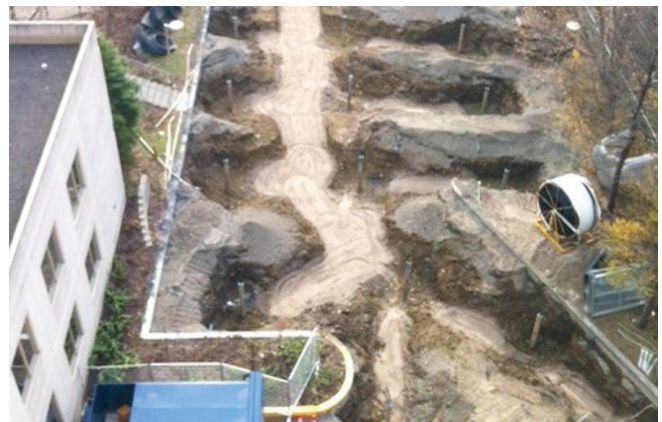
More than thirty wells were dug to sink piping for a new geo-exchange system at the Jewish Eldercare Centre, the second largest public Jewish long-term care facility in the Province of Quebec.
