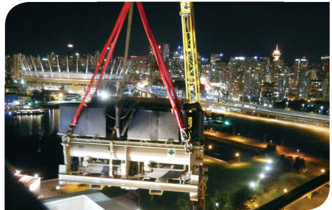
A 5,500 lb Trane® Series R™ Helical Rotary heat reclaim chiller, designed to boost the low grade heat generated from the centre, was hoisted to the rooftop mechanical room. Photo credit: Chris Goodchild/SES Consulting.
