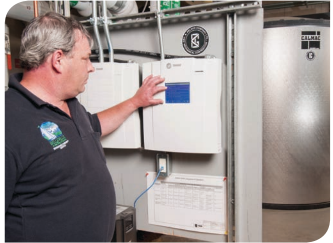
A Trane air-cooled chiller generates ice during off-peak utility rate hours. The system is controlled by the Trane Tracer Summit® building automation system.
