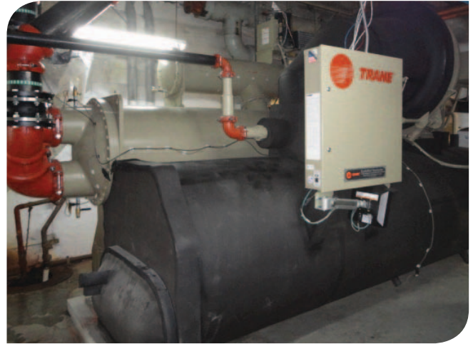
A 500-ton Trane high-efficiency CenTraVac centrifugal chiller with partial heat recovery helps reduce operating costs and provides reliable comfort for The Wave Condominium residents.
